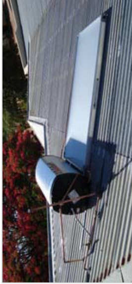
A Solar Water Heater uses energy from the sun to heat water for domestic use.
