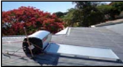
Solar Water Heater (SWH)
