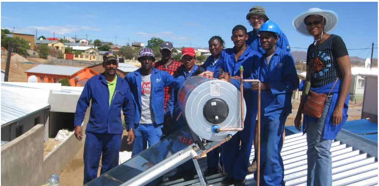
Installation of solar water heaters at houses in Otjomuise, Windhoek, built under the government mass housing initiative
