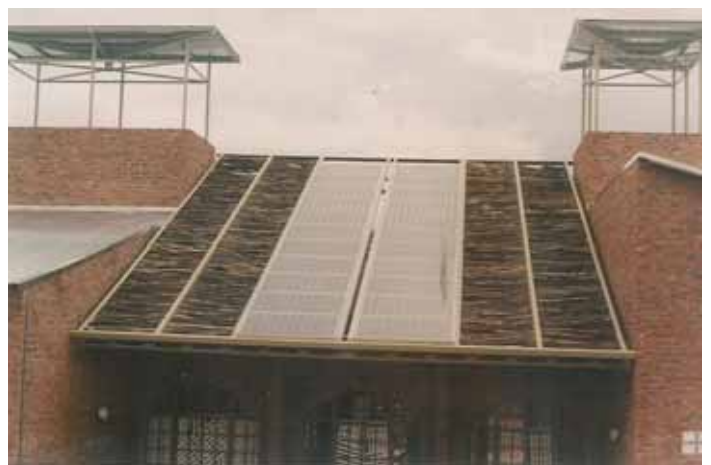
Photo-voltaic (PV) panels
