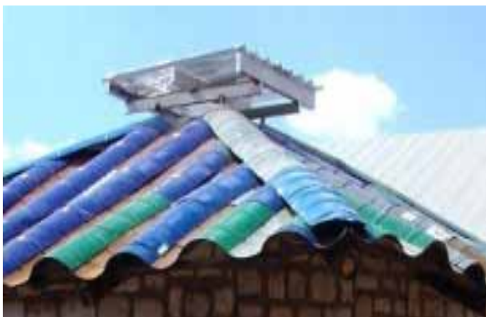
Passive Roof ventilation at HRDC.
